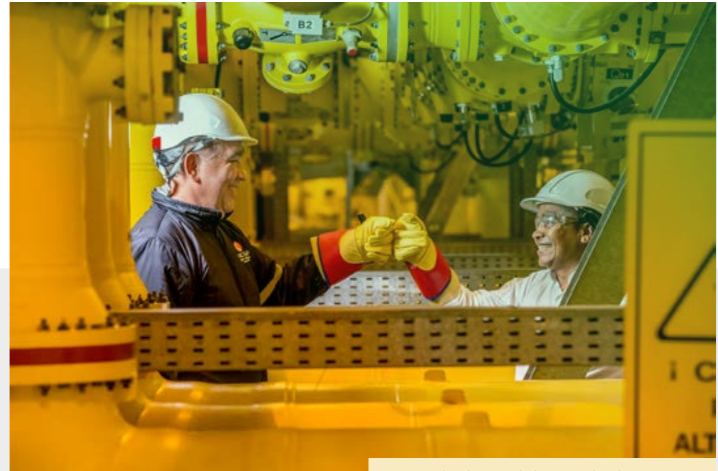
Guavio Transmission substation, Colombia
