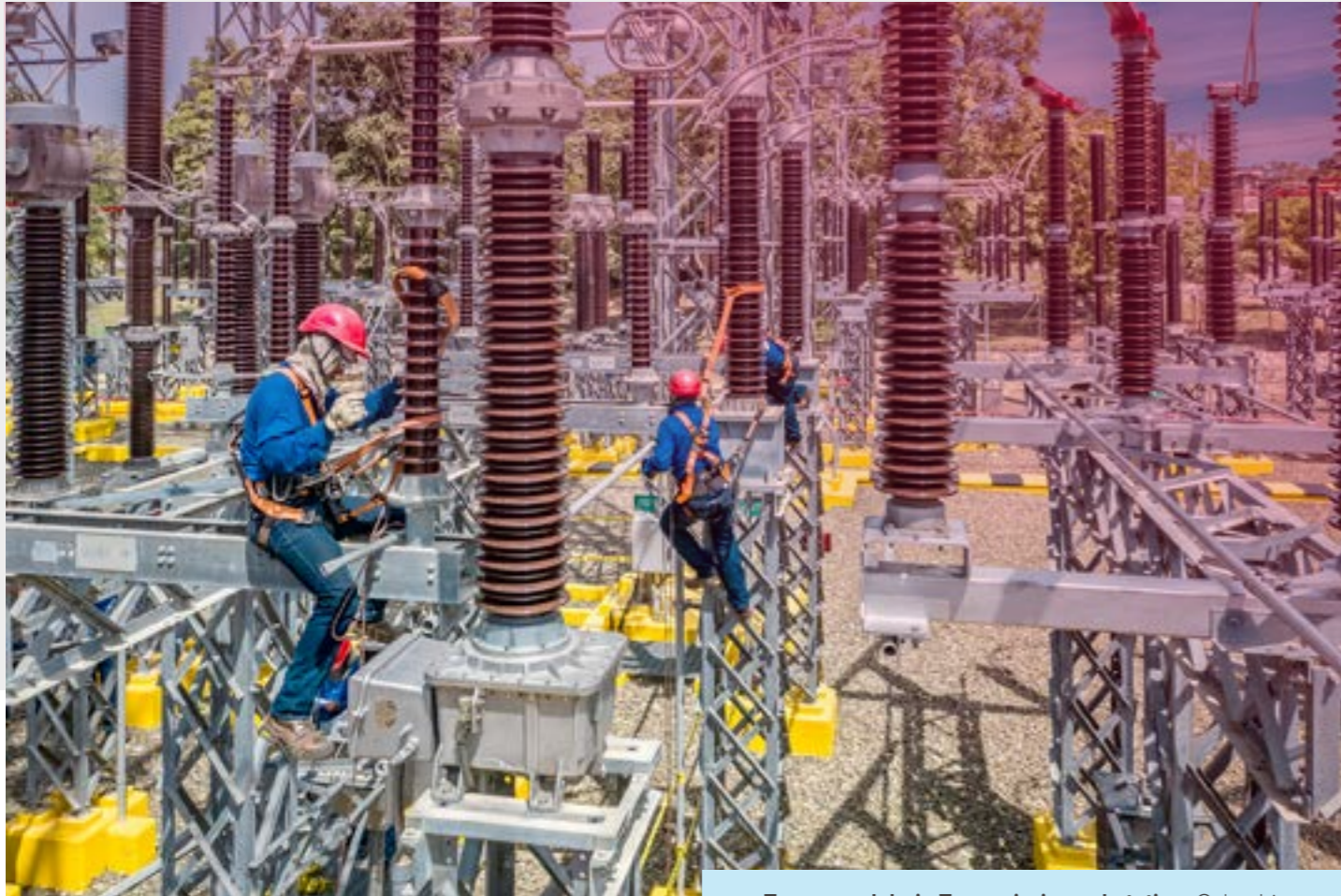
Termocandelaria Transmission substation, Colombia
