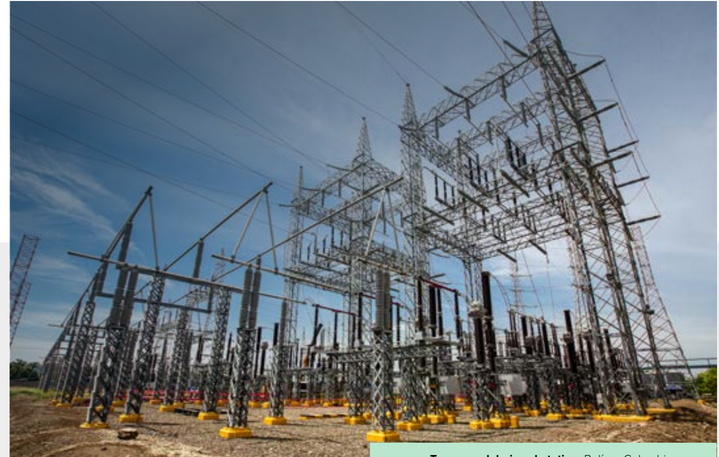
Termocandelaria substation, Bolívar, Colombia.
