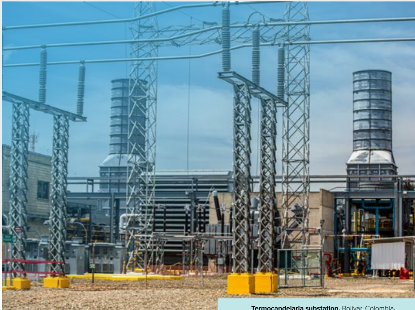
Termocandelaria substation, Bolívar, Colombia.
