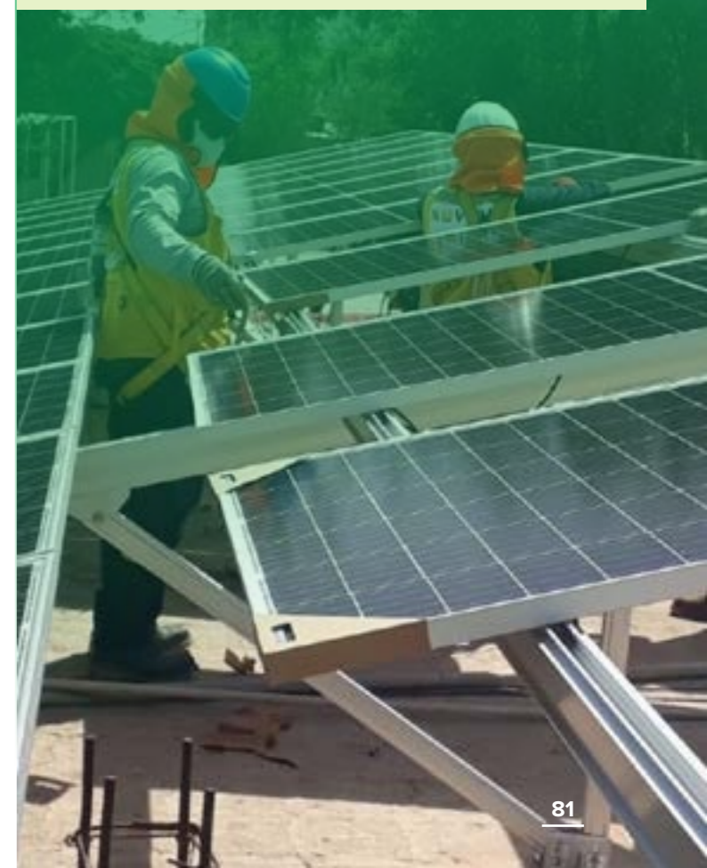
Solar panels at TGI La Guajira, Colombia.
