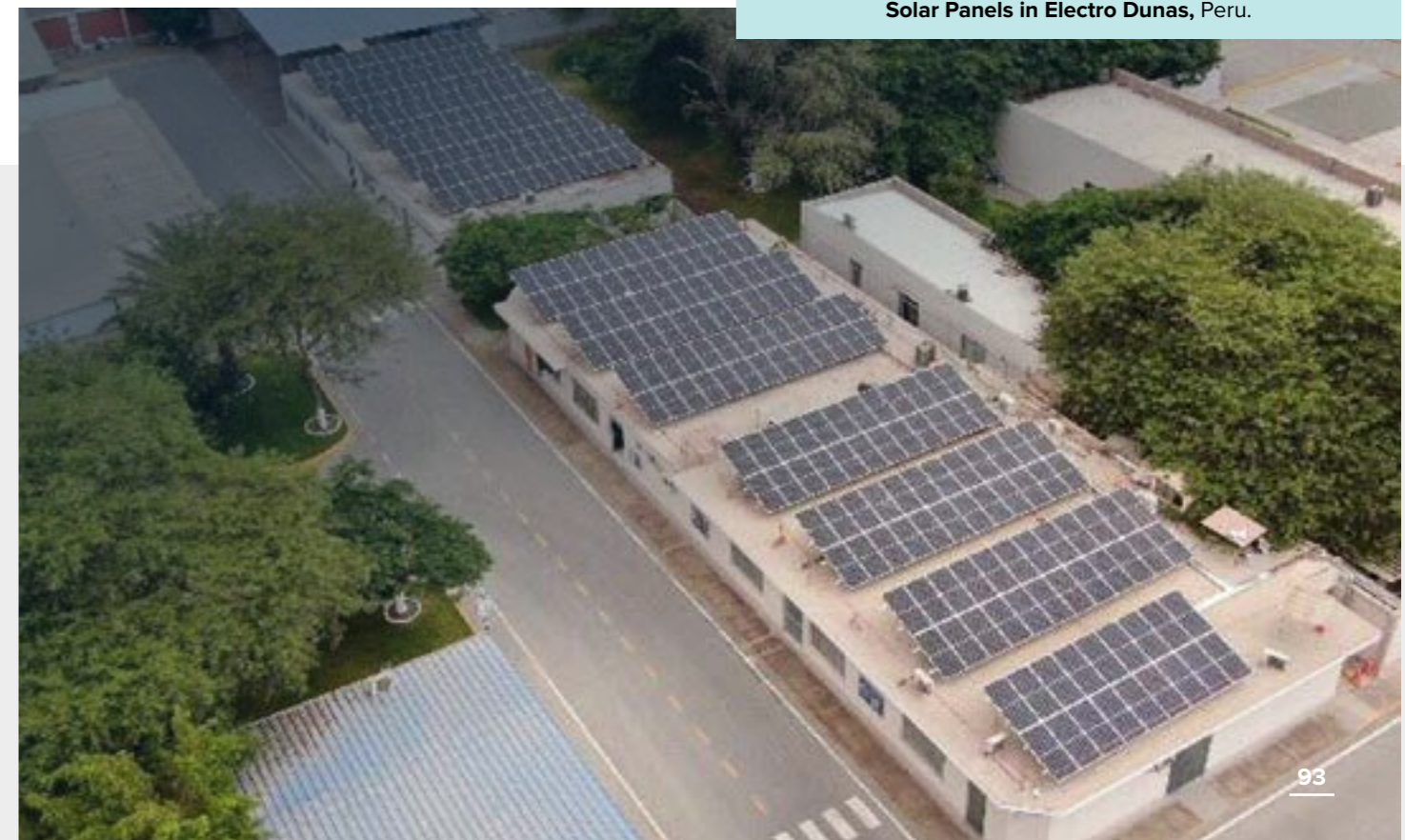
Solar Panels in Electro Dunas, Peru.
