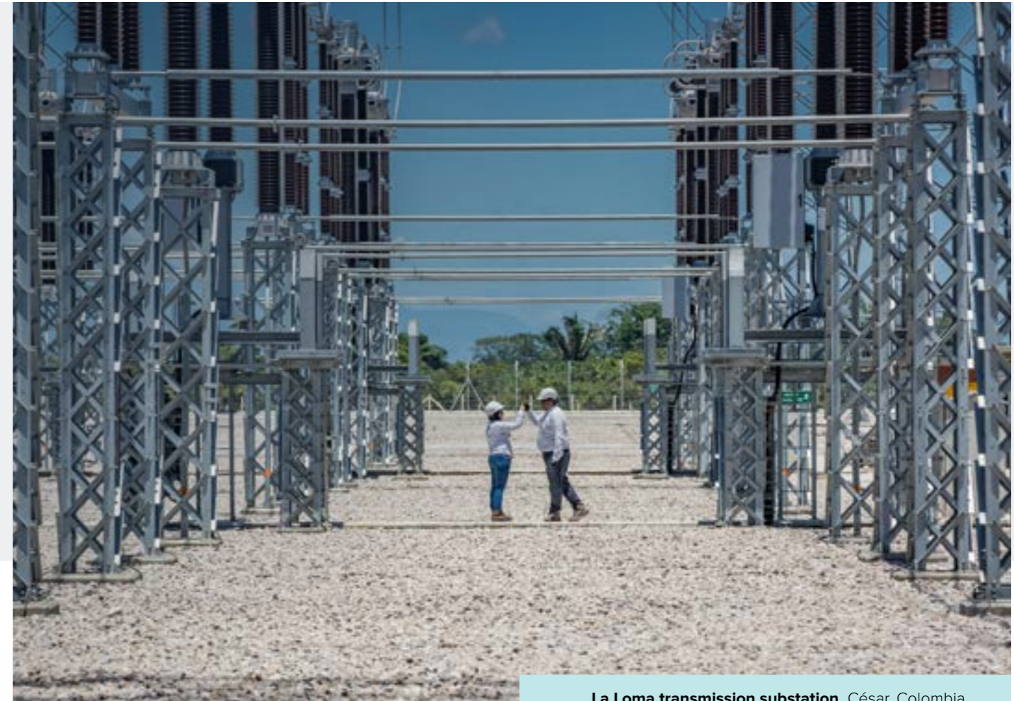
La Loma transmission substation, César, Colombia
