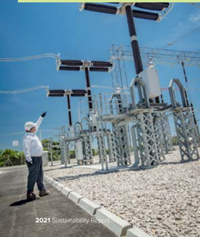
La Loma transmission substation, Colombia
