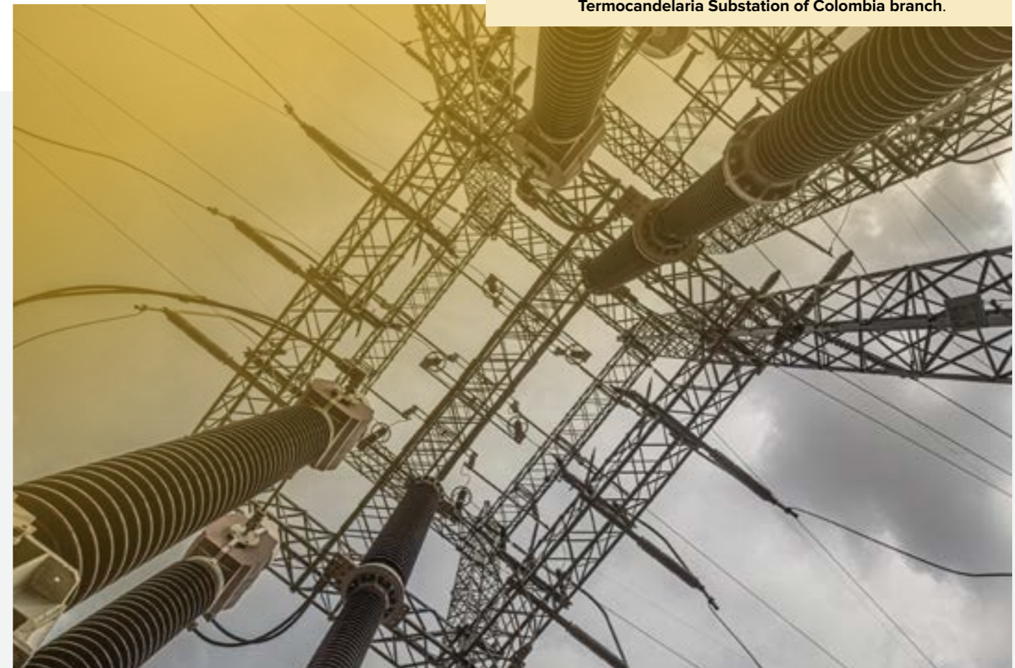
Termocandelaria Substation of Colombia branch.
