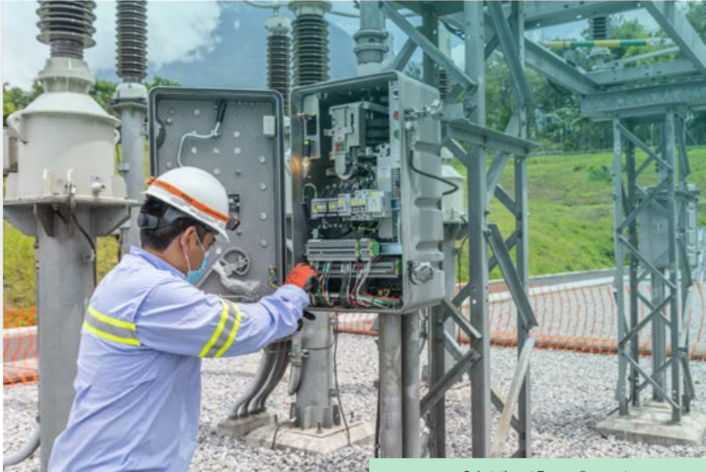
Substation at Trecca, Guatemala.
